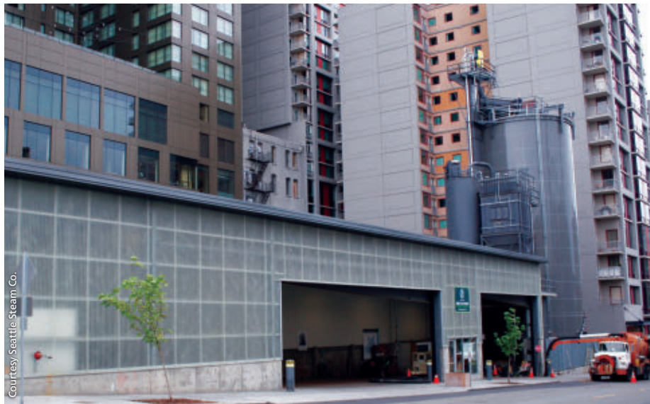
Seattle Steam’s new fuel handling facility is adjacent to one of its customers, the Four Seasons Hotel. The facility quickly took shape in 2009, with construction of the storage silo (right) attracting community attention. Uniquely, the roof section went up first, and the silo was built from the top down by jacking up each course of the tank over the eight-week construction time frame.
